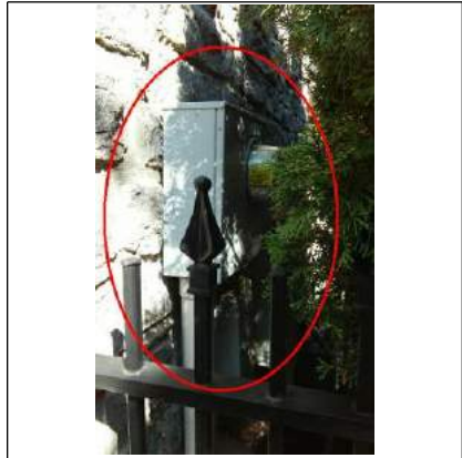
Service entry at left side facing.
