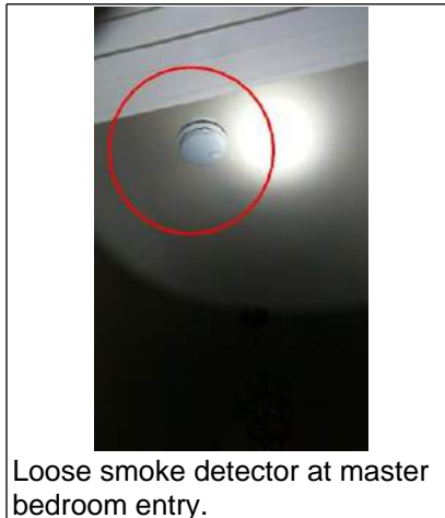
Loose smoke detector at second floor hallway.
