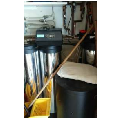
Water softener located in the garage closet.
